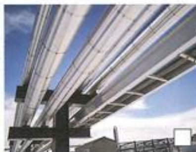
f pipe with hot oil inside
